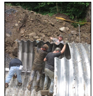
Assembly of plated arch pipe on Birdman Road Phase II, Quemahoning Township
