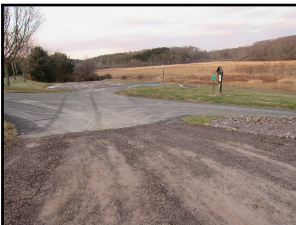
The reconstruction of the North parking lot is one of the first visitor improvements to the Somerset Lake Nature Park with more to come
