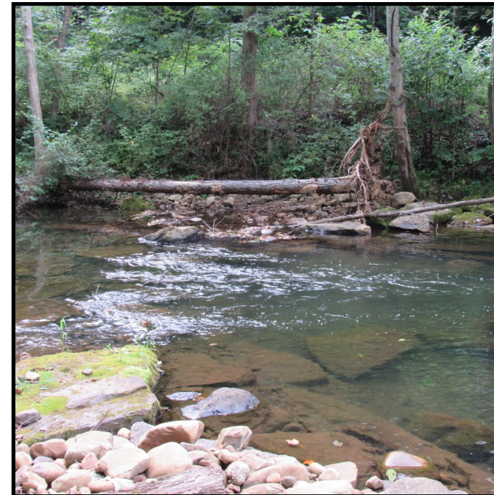
Rock and wood placement along with bank stabilization on the Que Tailwater.
